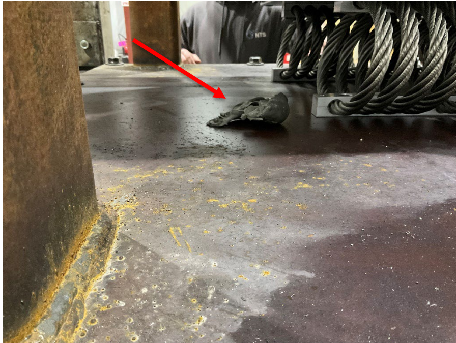
Photograph 5: Crushed Clay Cone – Right Rear Base Isolator
